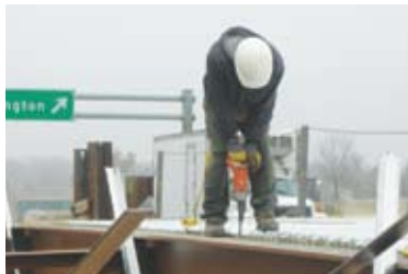
A worker secures deck pans for the widened southbound bridge in Fort Washington.
