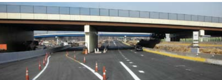
Considerable progress was made in 2007 on reconstruction of the southbound lanes at Fort Washington. PennDOT expects to shift traffic onto the new pavement, as shown here, in the first quarter of 2008.
