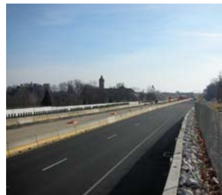
Southbound reconstruction between Willow Grove Avenue and Easton Road was completed in 2007.
